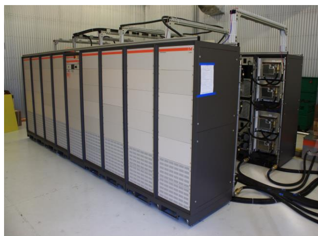
Figure 1. HF Amplifier installed in the REG
